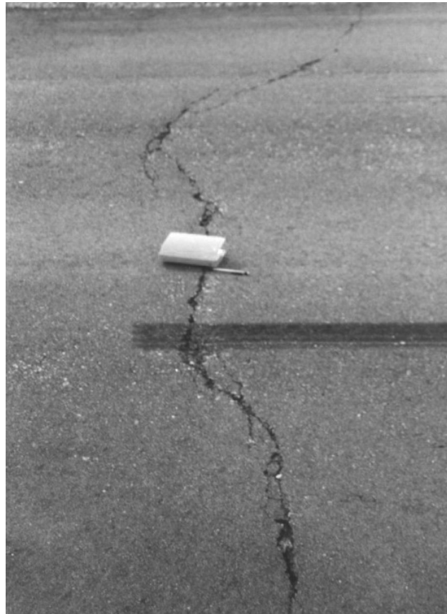
Figure 4 Surface Cracking at a Pipeline Crossing
