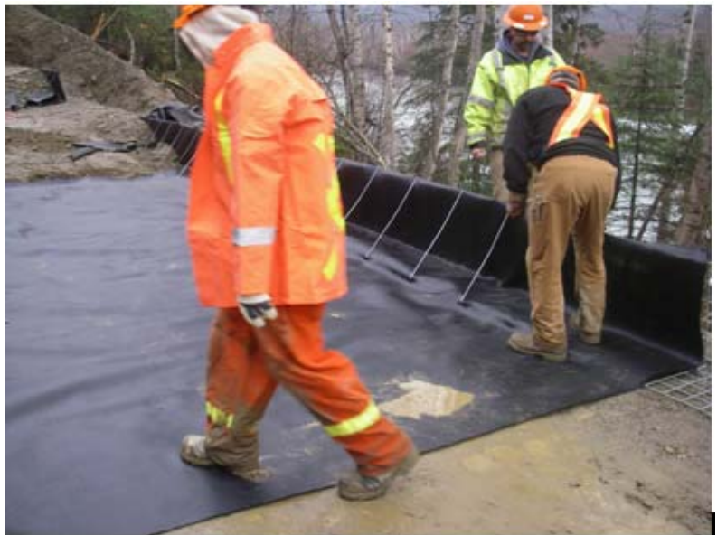
Figure 2 – Poser Siding: Wall 1 View Showing Assembly of GRS Facing and Fabric System.
