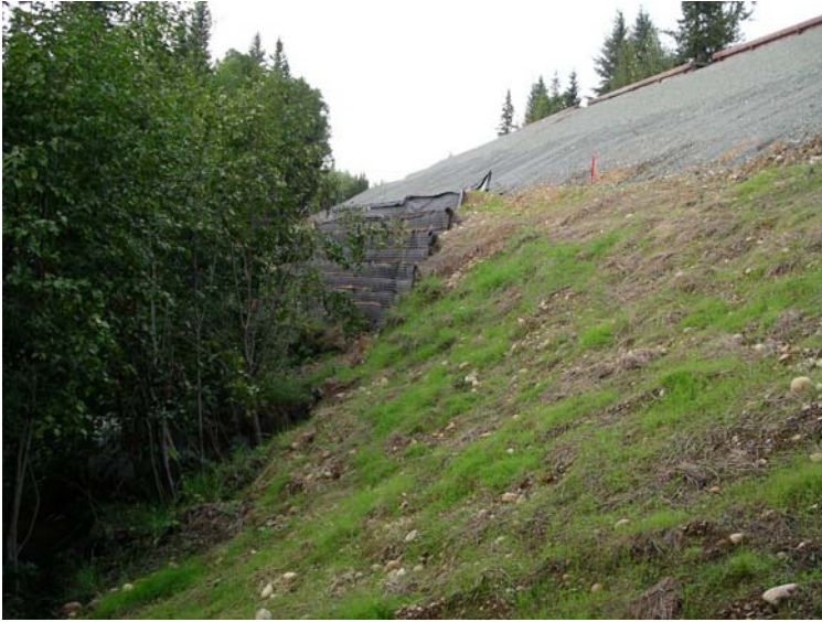
Figure 13 – Matheson Siding: Bittner Creek. View Looking Track-south at Completed Wall Illustrating how the Wall Blends into the Standard Fill Slope Section.
