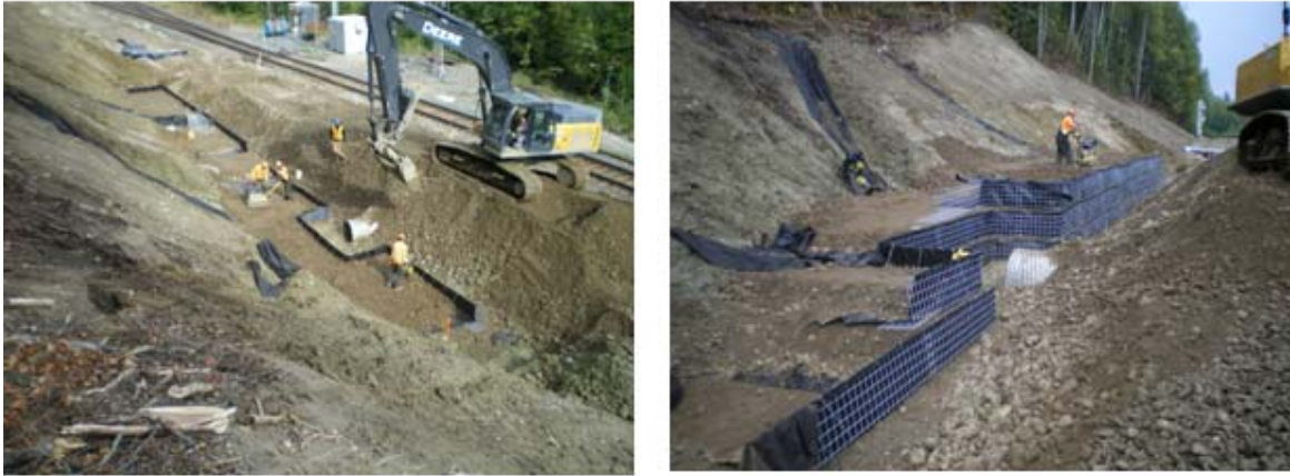
Figure 7 – Poser Siding Wall 5. Views Showing the Flexibility of the Wall System to Incorporate French Drains and Culvert Inlet Basins.
