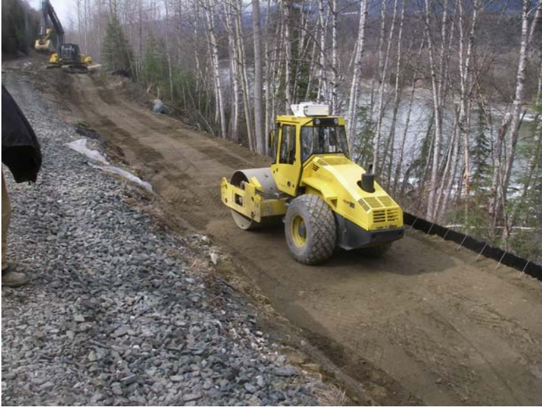
Figure 3 – Poser Siding: Wall 1 View Looking Track-north During Construction Showing Compaction of Fill.
