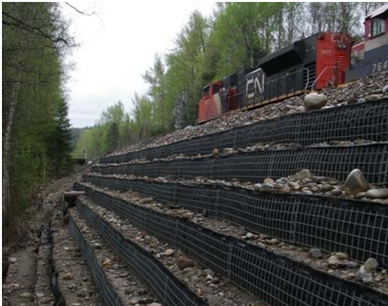
Figure 4 – Poser Siding: Completed Wall 1 Looking Track-south. Note Culvert Extension Built Into Wall.
