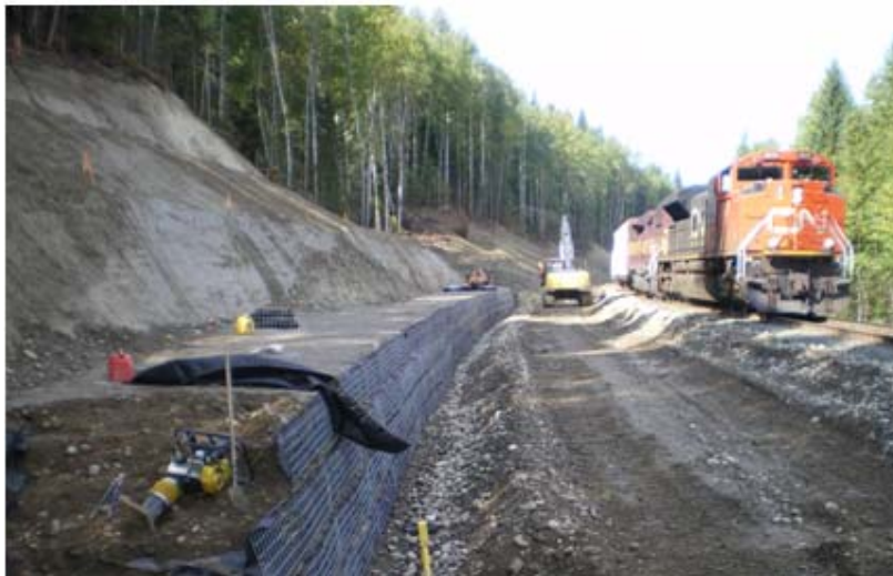
Figure 8 – Poser Siding Wall 5. View Looking Track-north Showing Temporary Cut, Wall Construction, Construction of New Grade, and Existing Grade. GRS Beneath New Grade has not yet Been Placed.
