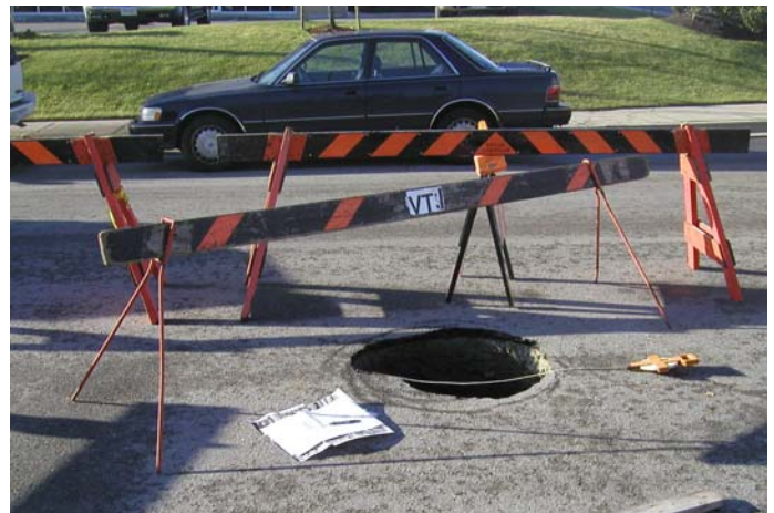
Figure 4. Photograph of a sinkhole in Coquitlam, B.C.
