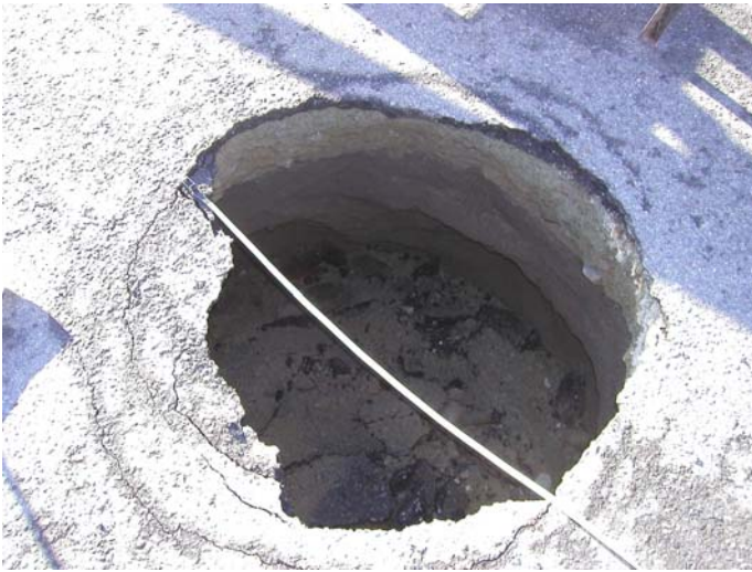
Figure 5. Photograph illustrating the vertical nature of the sinkholes observed in Coquitlam, B.C.
